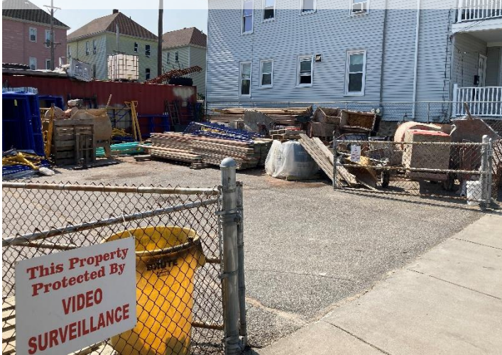
Material and equipment are stored along the property line. Looking southwest from Howard Avenue.
